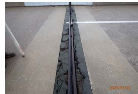
Image 6: Multiple failing deck joints with full depth spalls
