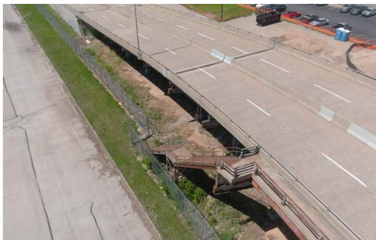
Image 4: Existing deteriorated staircase with no adjoining pedestrian path
